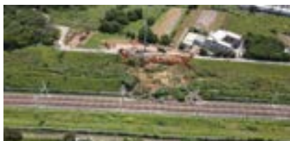
Slope failure stage and collapse range
